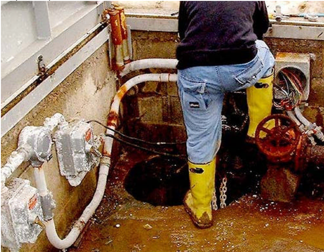
Fig 1. Jeff prepares to enter the ground pit. White corrosion on the wiring is caused intermodulation fumes from the link repeater.
